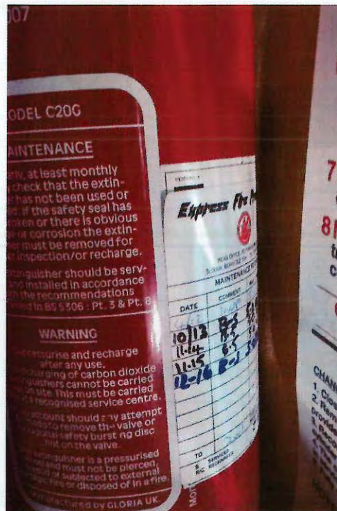
17. Fire extinguisher within basement.
